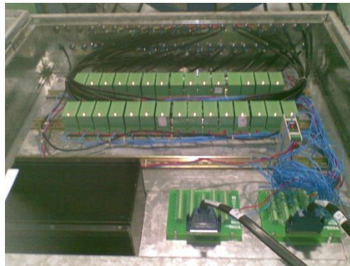
signal conditioning box
